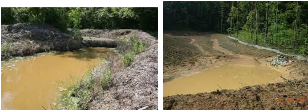
Figure 9: Typical Silt Trap/Settlement Pond Installations
